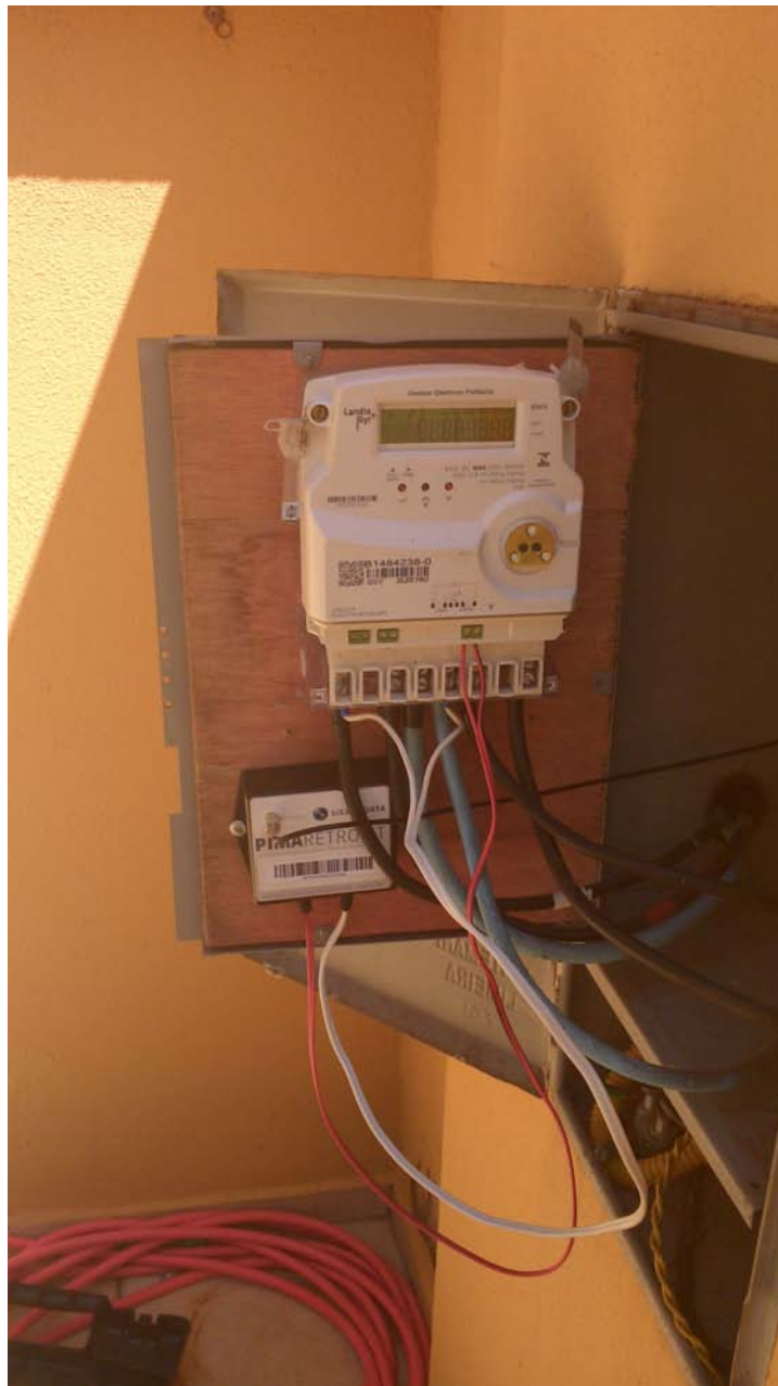
Figure 4. CyLec retrofit solution deployed in Brazil
