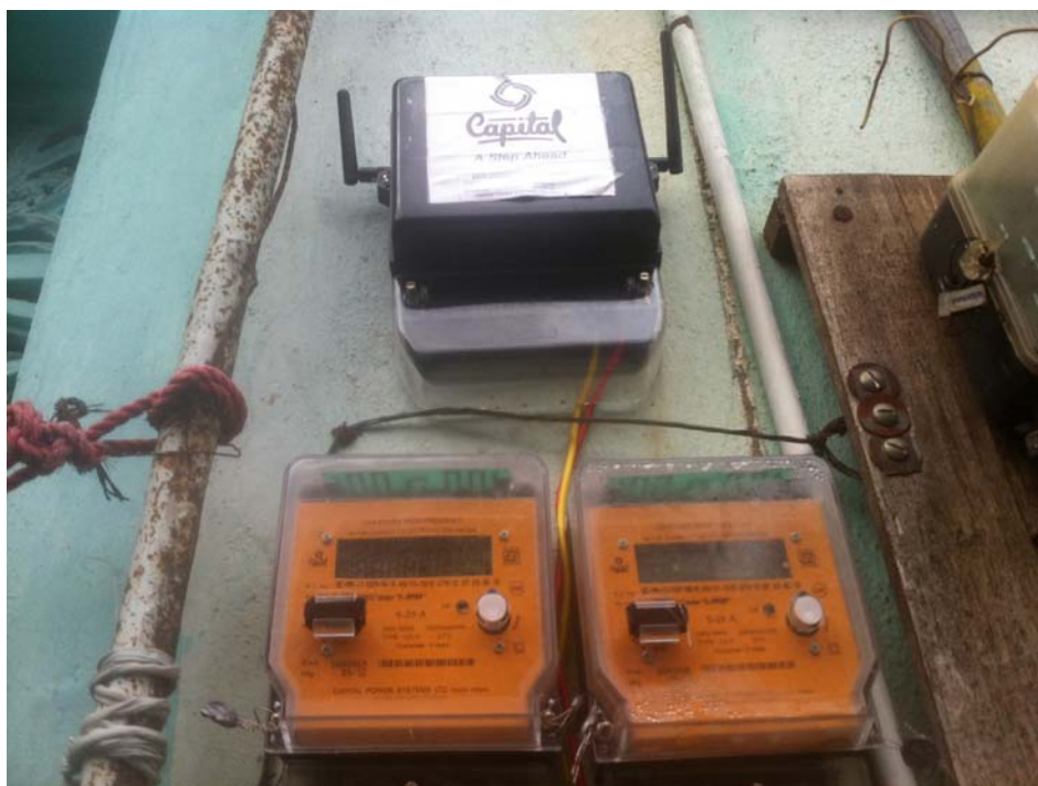
Figure 3. CyLec enabled meters deployed in Trichy, Tamil Nadu, India
